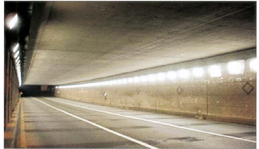
After Induction fixtures 100 W
