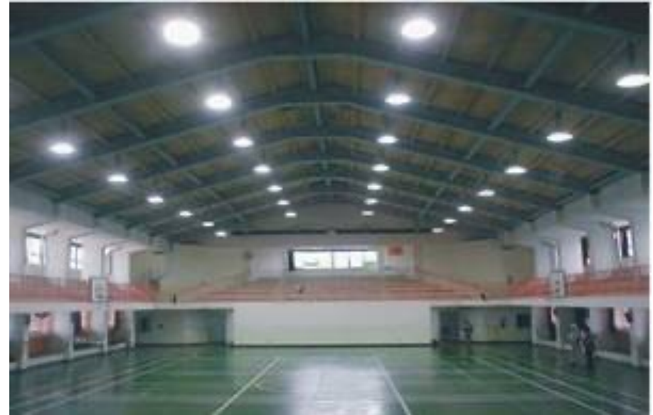
After Induction Fixtures 100 W
